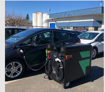
Mobi is ideal for fleet locations where there is little or no electrical infrastructure available to support fixed charging
