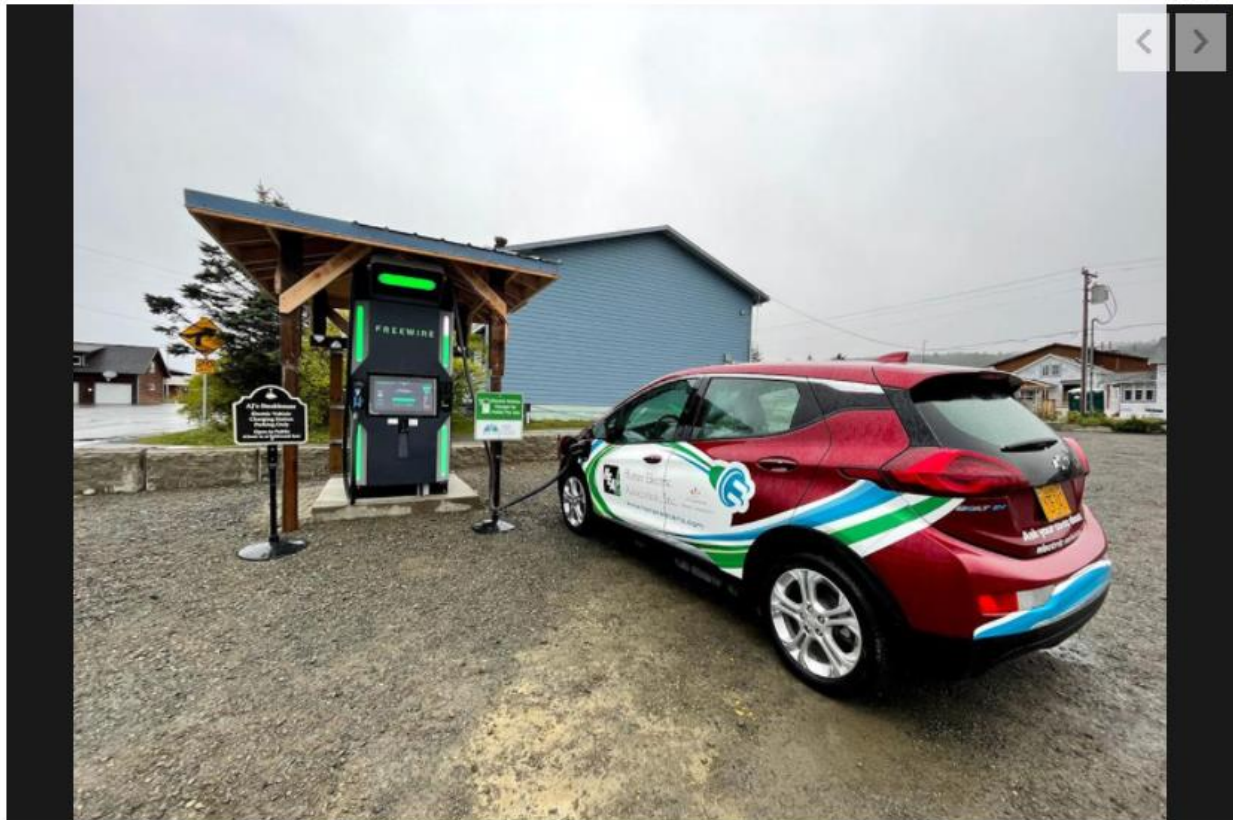
An electric vehicle plugs into the fast-charging EV station, developed by FreeWire Technologies of California. The station can accommodate two vehicles at a time. ALL PHOTOS COURESTY OF Jorden Perez, Kachemak Communications Jorden Perez, Kachemak Communications
